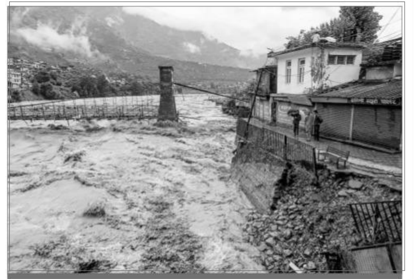
Damaged Bhuntar Valley Bridge after a section was washed away in the swollen Beas river owing to incessant monsoon rainfall, in Kullu district, Monday, July 10, 2023.
