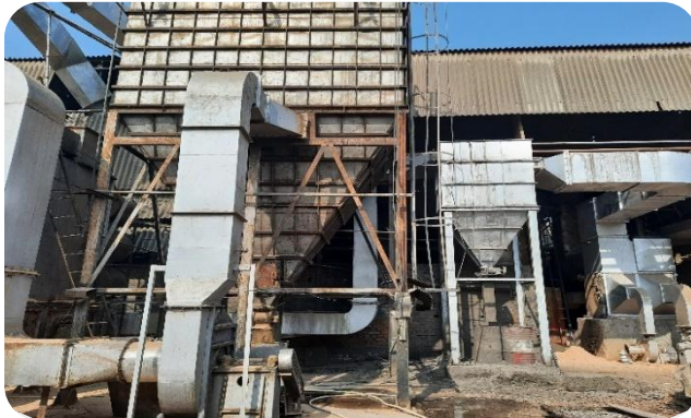
Thermic Fluid Heater
