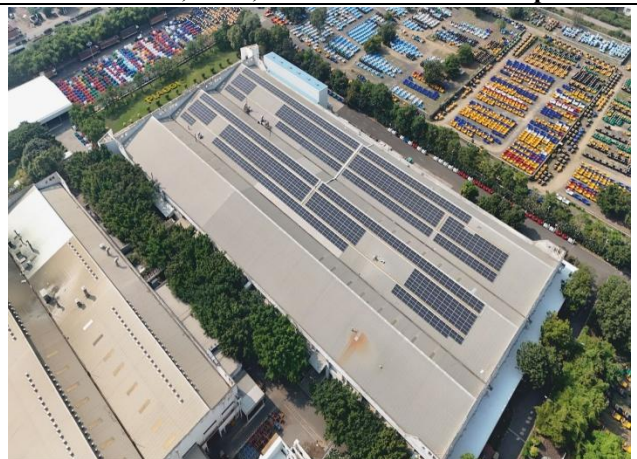
Baramati, Pune, Maharashtra - 1000kWp
