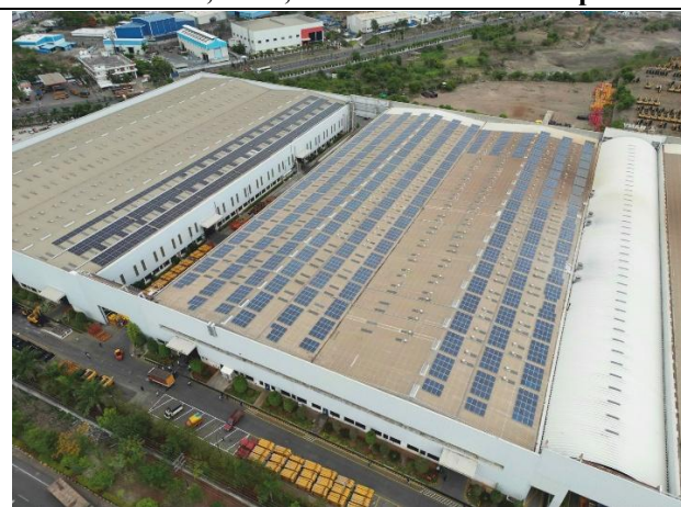
Chakan, Pune, Maharashtra - 400 kWp
