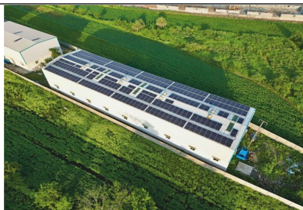
Chakan, Pune, Maharashtra - 120kWp
