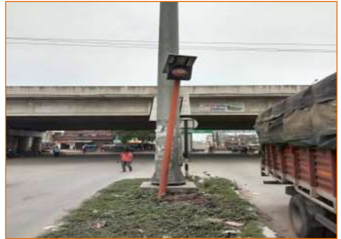
LED Blinker at km. 754+441
