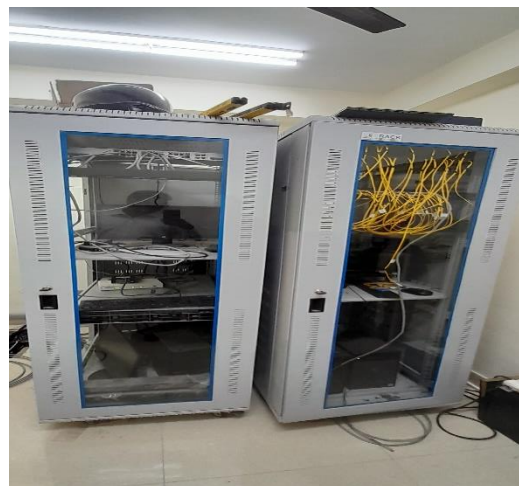
Figure 9-12 Control Room Equipment - Server & Switch rack
