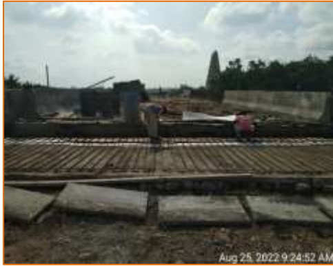
Approach slab work @ A2 side of Flyover is in progress at km. 136.857 (LHS)
