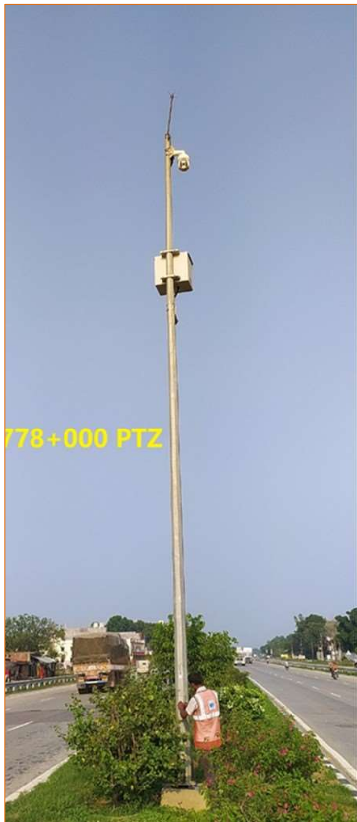
Figure 9-9 PTZ camera at km. 778.000
