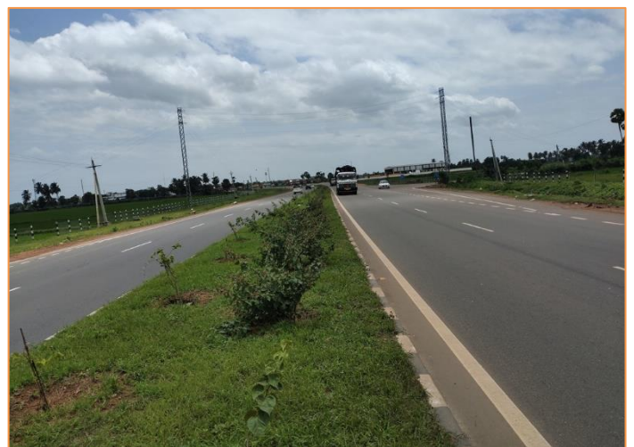
Pavement Condition at km. 57+200
