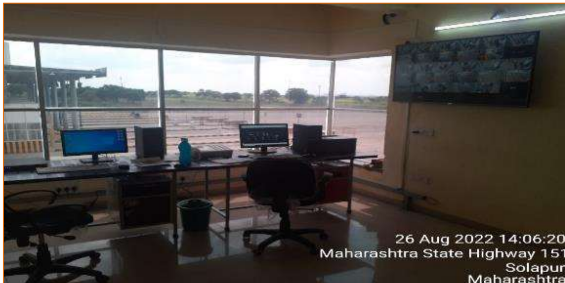
Figure 9-10 Incident Management Workstation at Control room
