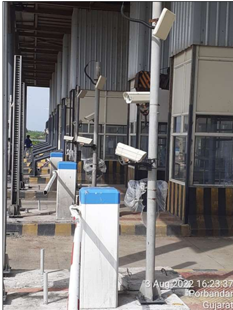
Figure 9-3 RFID ETC Reader mounted on Pole
