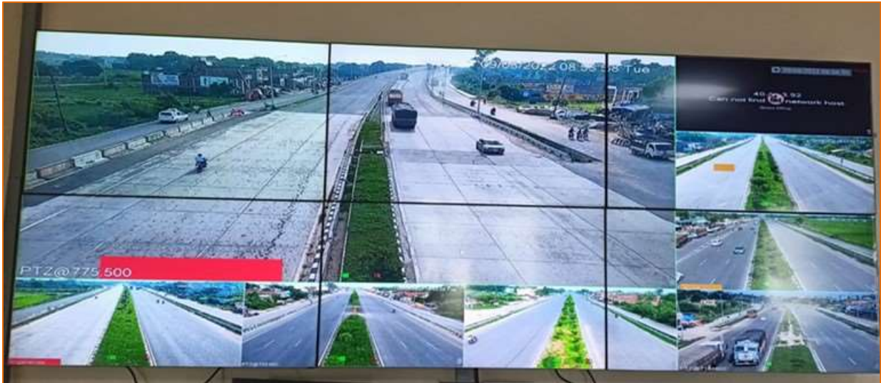
Figure 9-10 Video wall in ATMS control centre
