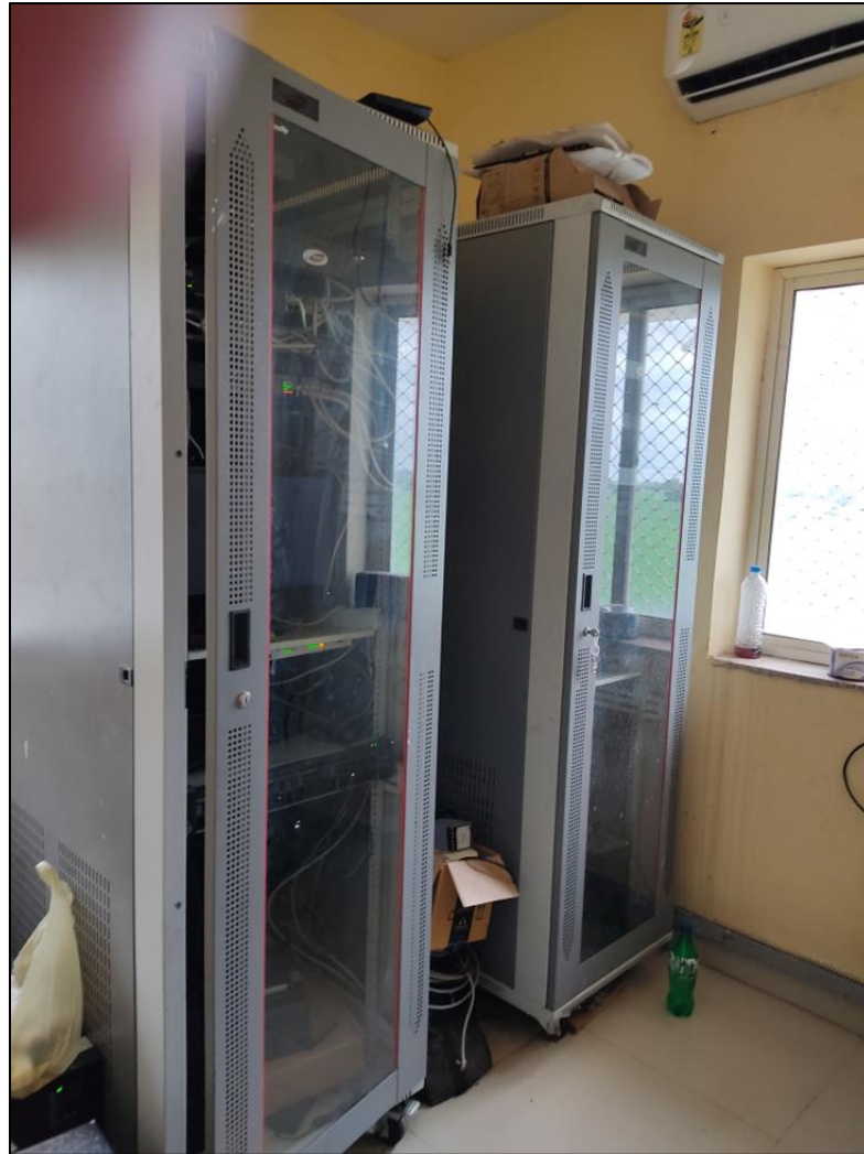
Figure 9-13 Control Room Equipment - Server & Switch rack
