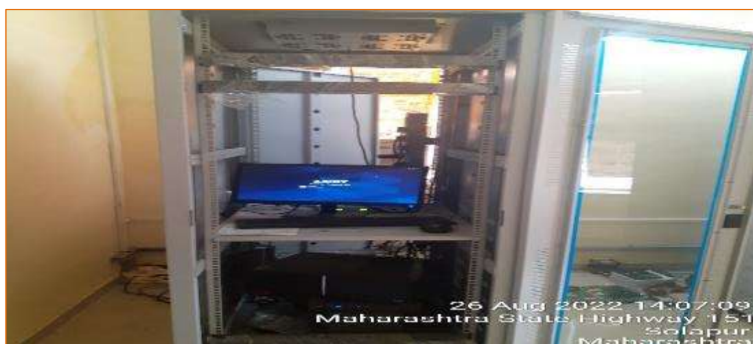
Figure 9-8 Medium Control Room Equipment – Server & Switch rack
