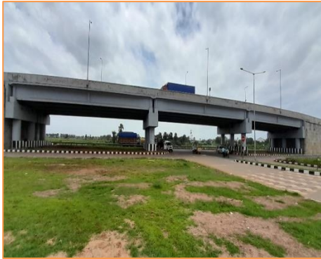
View of UDFO at km. 15+800
