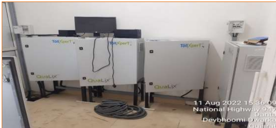
Figure 8-3 Lane Controllers for normal ETC lanes
