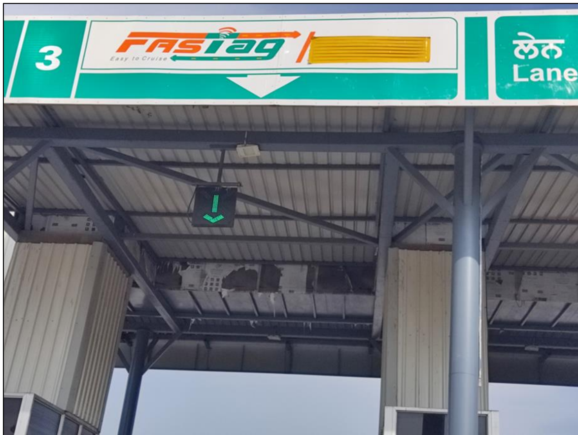
Figure 9-10 Over Head Lane Signal (OHLs)
