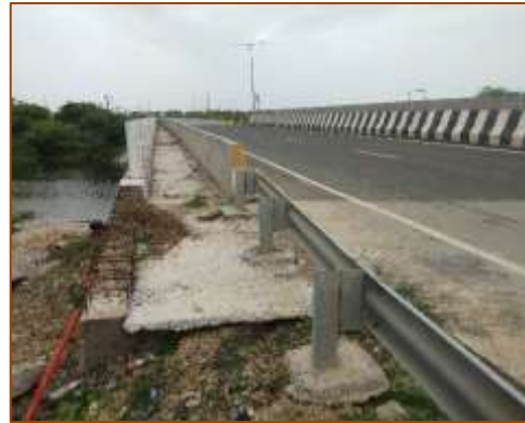
Return wall beam bending of MNB at km. 456+533 (RHS)
