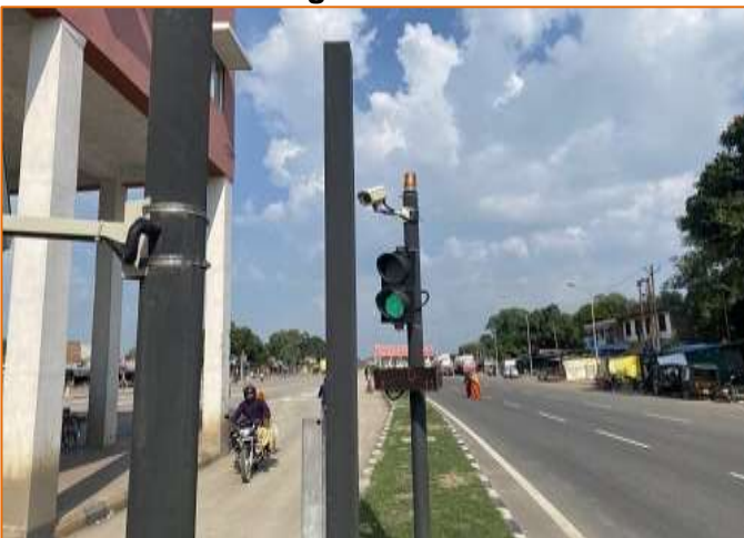
Toll Signal light
