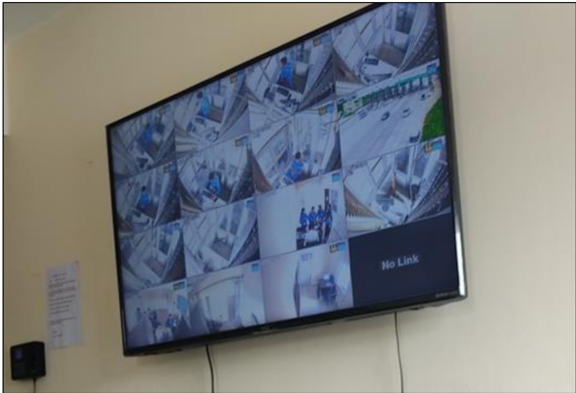
Figure 9-14 CCTV screen at the Toll Plaza Control Room
