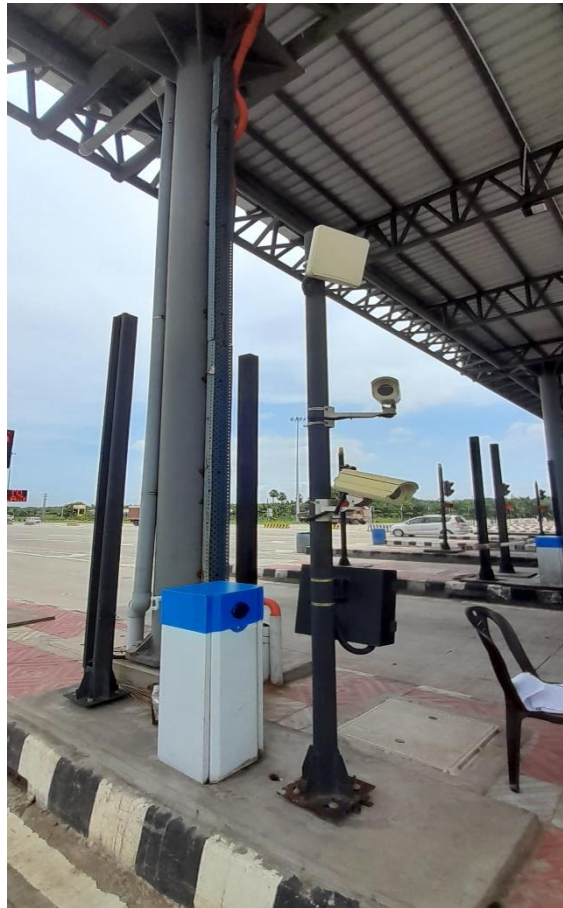
Figure 9-2 RFID ETC Transceiver installed on pole
