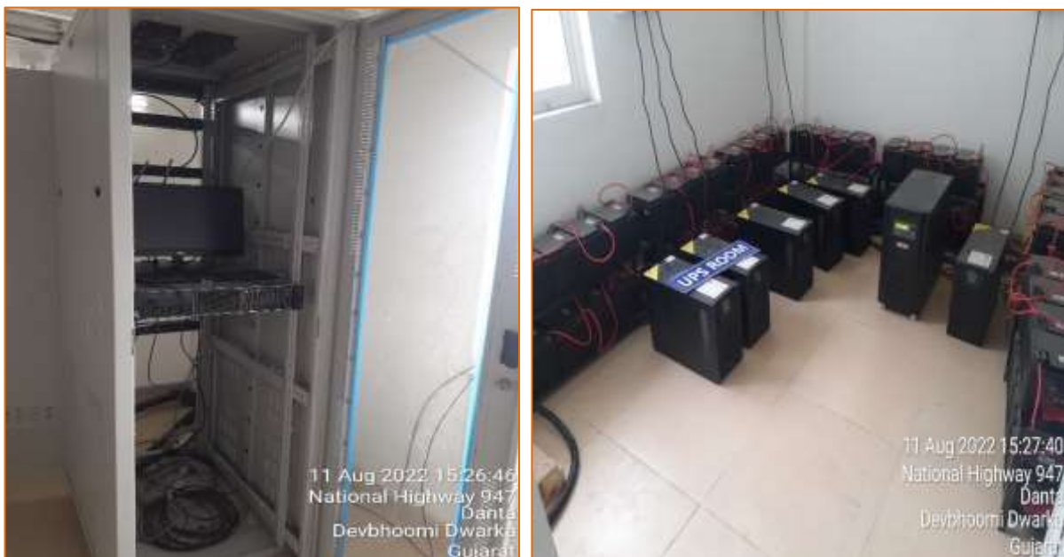
Figure 8-8 Control Room Equipment - Server & Switch rack/UPS Room
