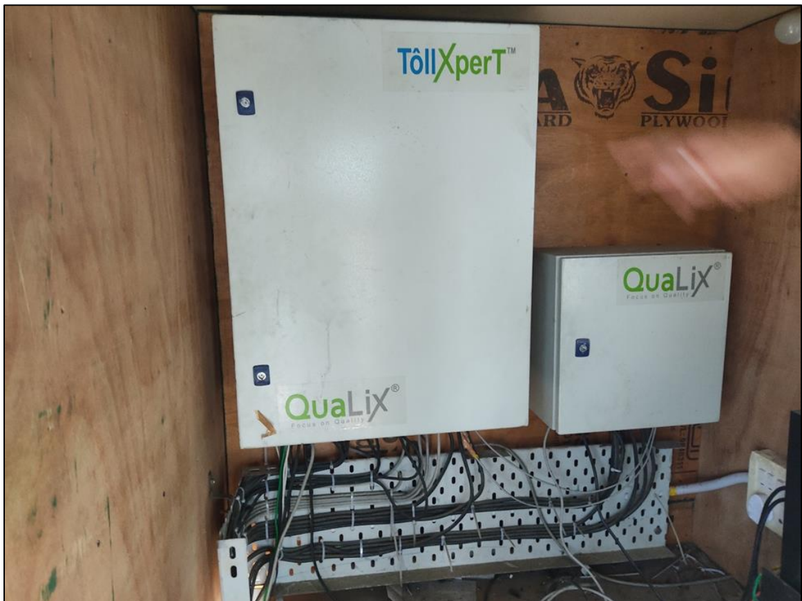
Figure 9-4 Lane Controller and AVC installed in enclosures at Toll Booth
