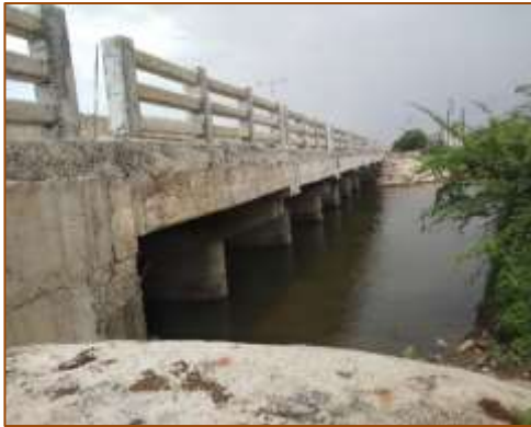
Side View of Minor Bridge at km. 455+195 (LHS) - Missing railing
