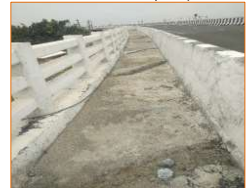
Uneven Drain with footpath at A1 side of MJB at km. 422.314 (LHS)
