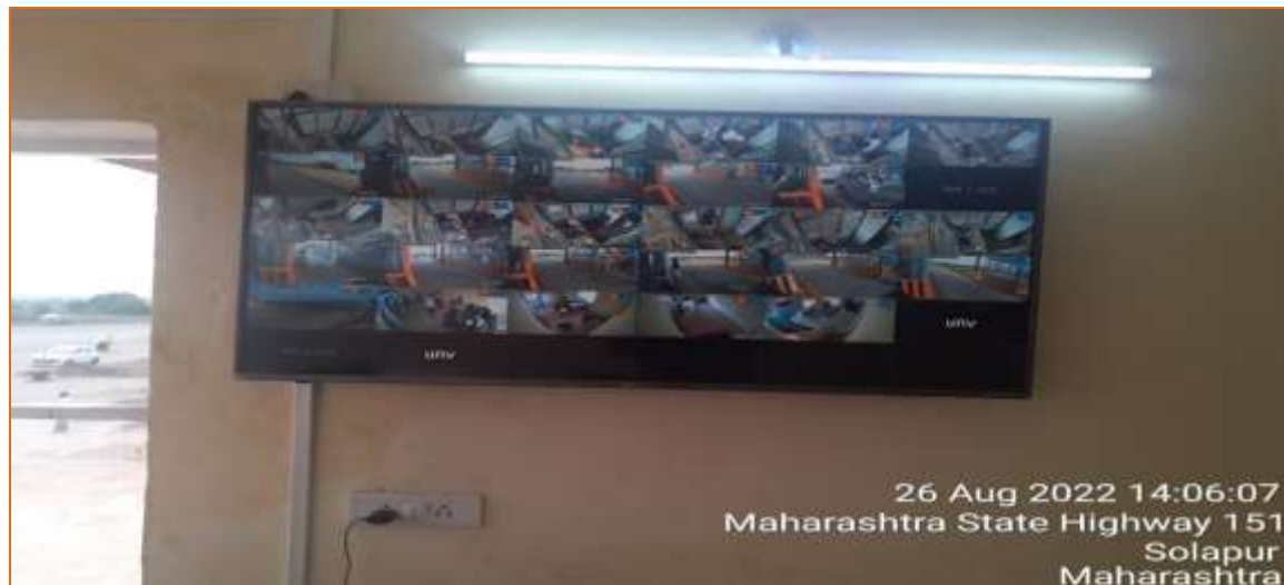
Figure 9-9 CCTV screen at the Toll Plaza Control Room
