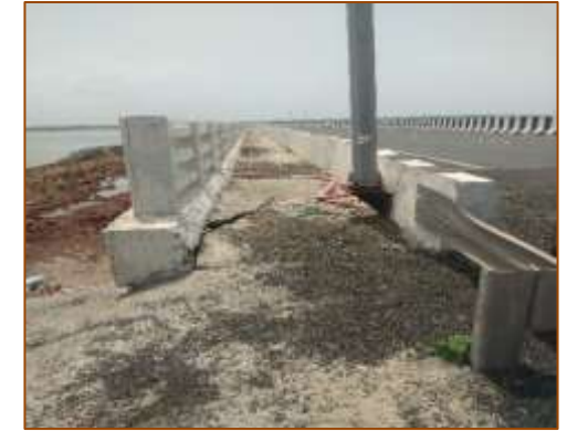
Major Bridge - km. 433+295 (RHS) Footpath settled
