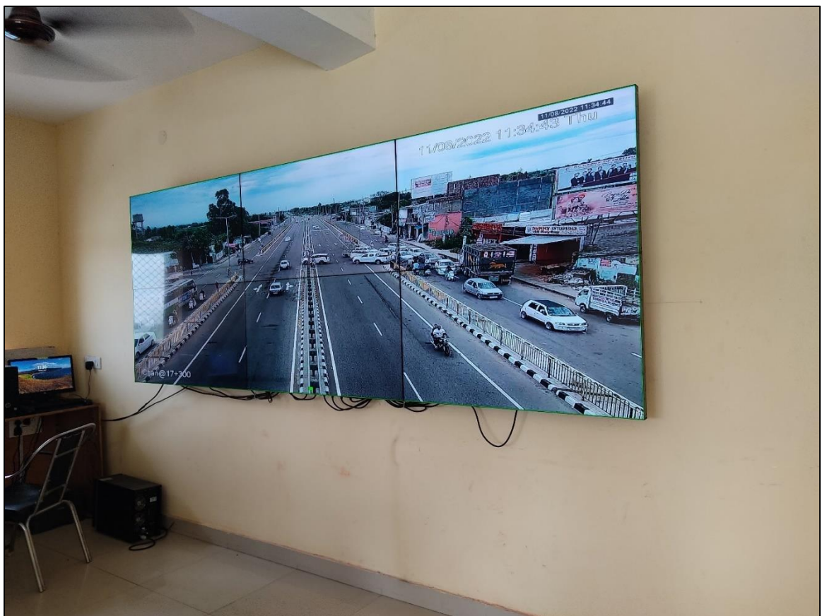
Figure 9-18 Video wall at HTMS Control room
