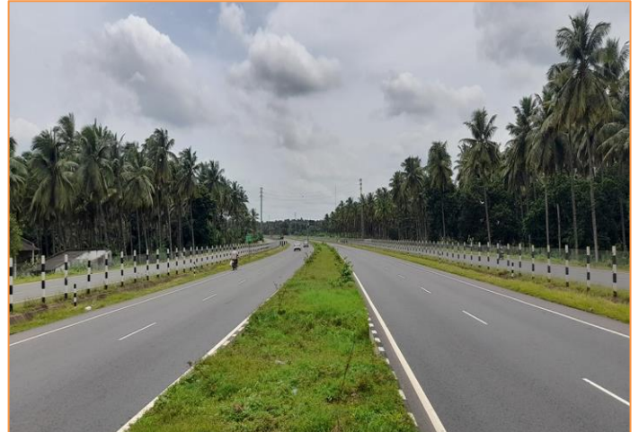
Pavement Condition at km. 46+700
