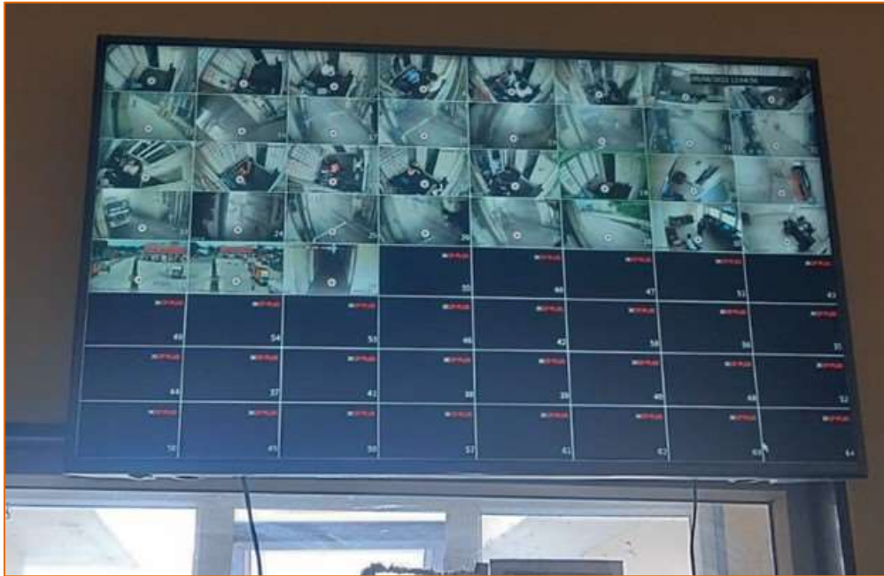
Figure 9-5 55" LED screen for CCTV monitoring
