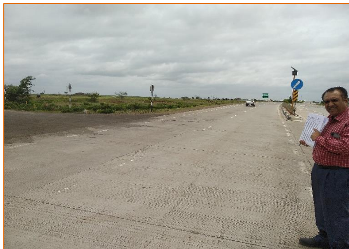
Pavement Condition at km. 306+500 (LHS)
