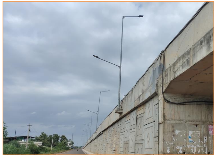
Highway Lighting at km. 44+135
