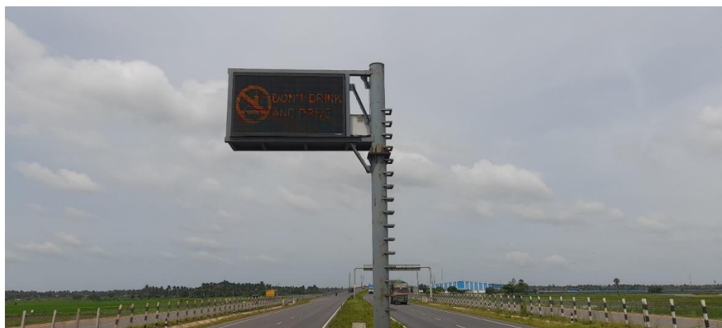
Figure 9-16 VMS on project highway
