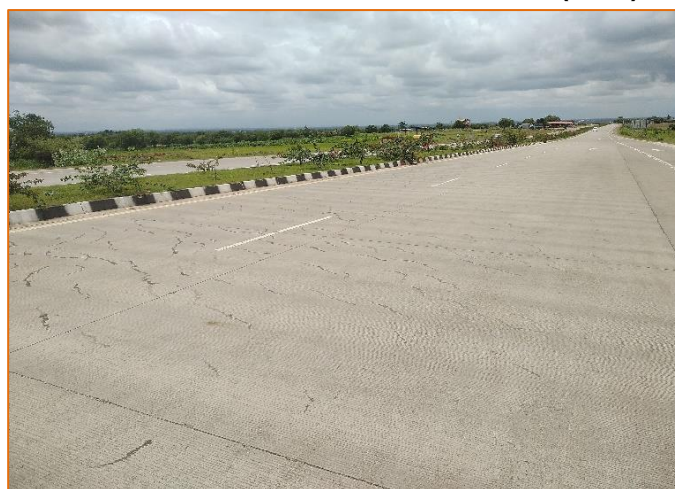
Pavement Condition at km. 304+600 (LHS)
