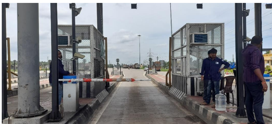
Figure 9-6 Automatic Lane Barrier
