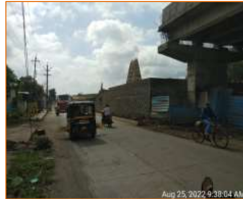
RE Block wall & FSCB of Flyover pending at km. 136.857 @ A1 side (RHS)
