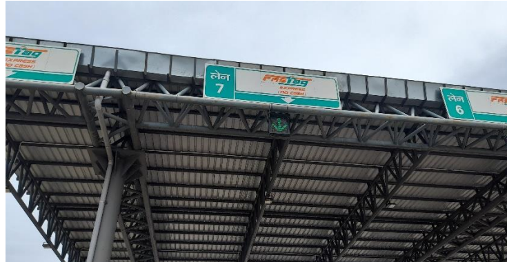
Figure 9-9 Over Head Lane Signal (OHLS)
