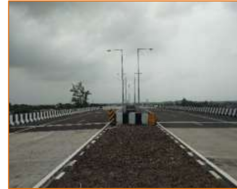
Wearing Coat of VUP (Limdi) at km. 23+120 (BHS)
