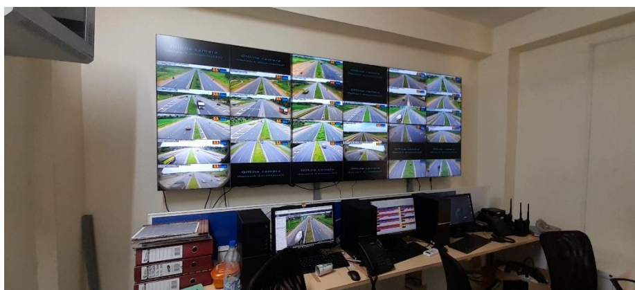
Figure 9-17 Video wall at ATMS Control room
