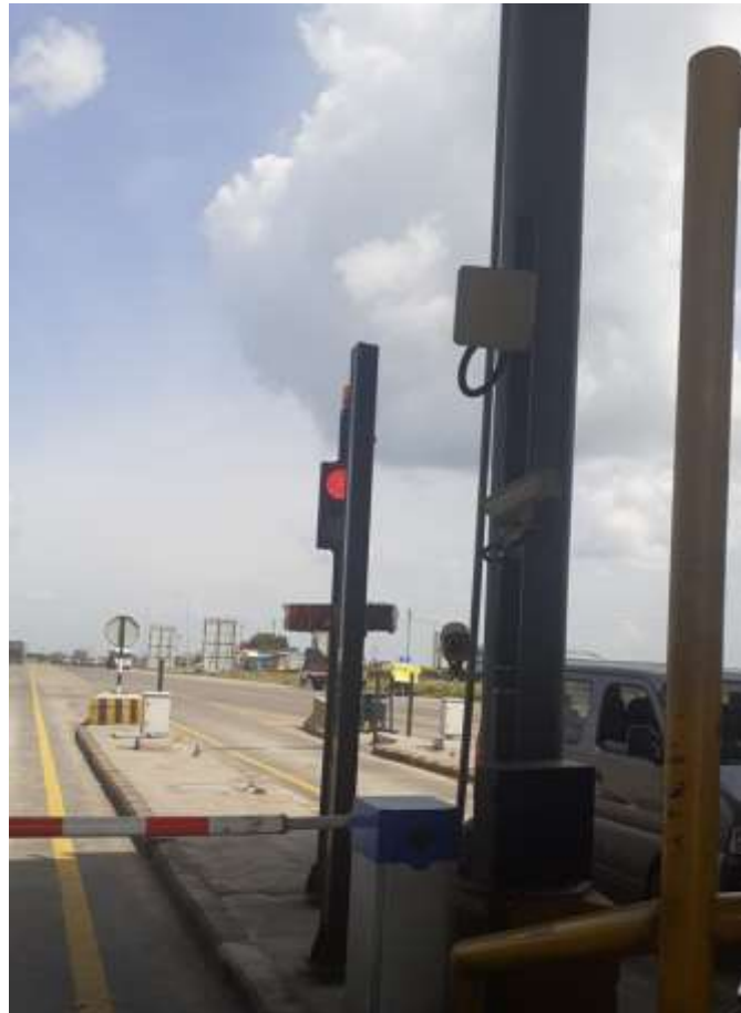
Figure 9-2 RFID ETC Reader mounted on Pole
