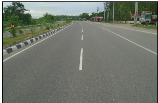
Pavement Condition at km.75+000
