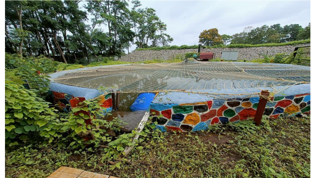
UG open Tank Capacity - 1 Million Litres
