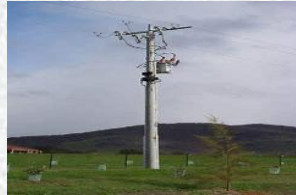
Power Distribution Poles
