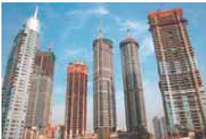
HVAC services for Omkar Realtors & Developers, Mumbai
