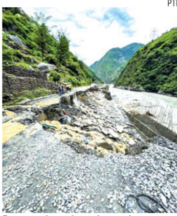
Damaged portion of a road following heavy rainfall in Chamba
