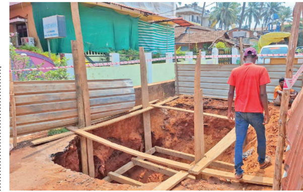
Calangute sewerage project has still not been tarred," he said, adding that the latest digging work was unlikely to be completed before the onset of the monsoon.
