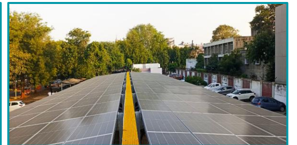
140 KW car parking solar for GSFC 2
