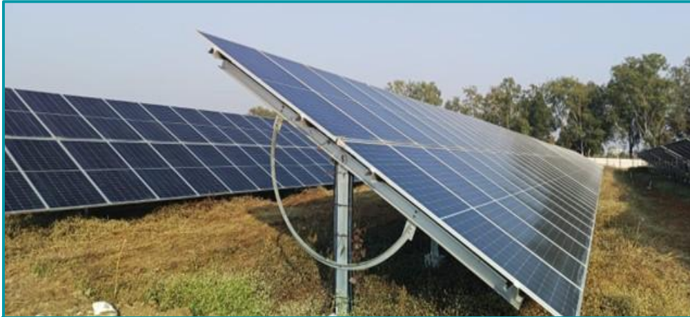
10 MW utility solar for multiple clients*
