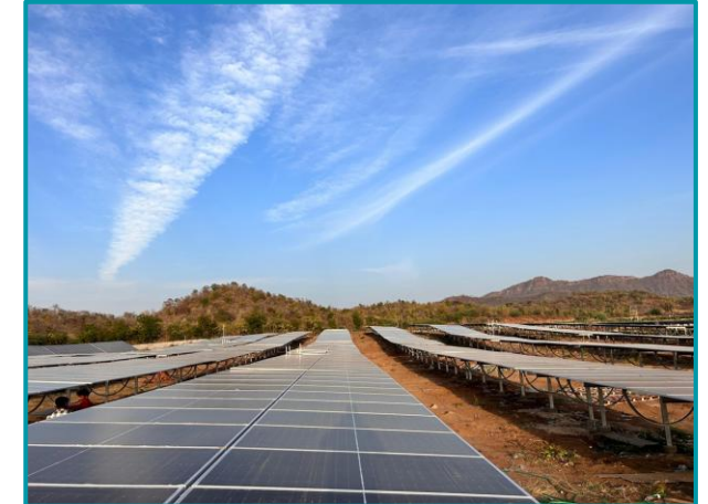
12 MW utility solar for multiple clients
