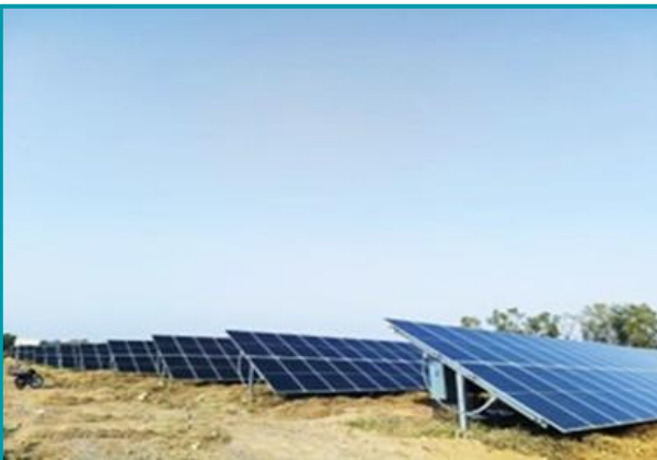
2.5 MW utility solar for GIFT Power Company
