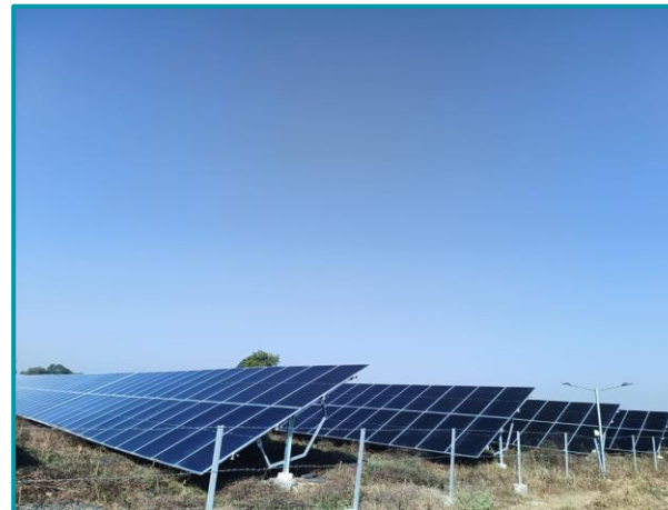
11 MW utility solar for multiple clients
