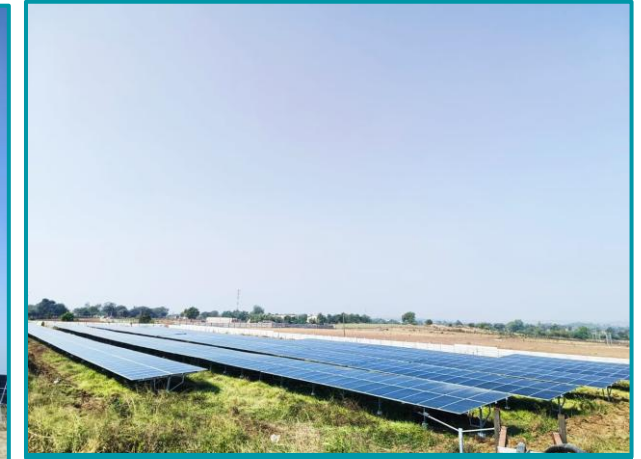
5.2 MW utility solar for Shivam Steelcast
