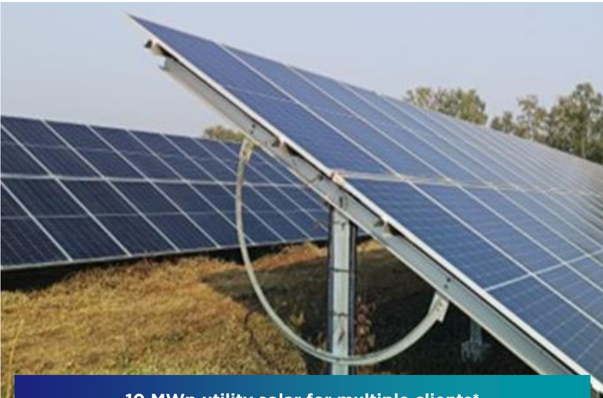
10 MWp utility solar for multiple clients*
