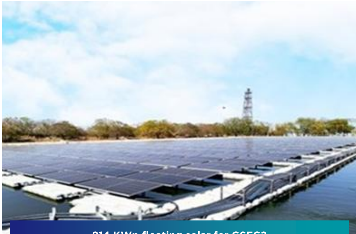
814 KWp floating solar for GSFC2
