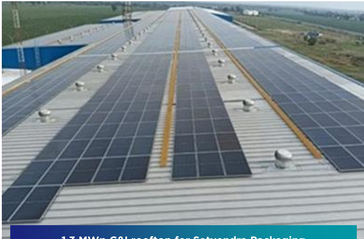
1.3 MWp C&I rooftop for Satyendra Packaging
