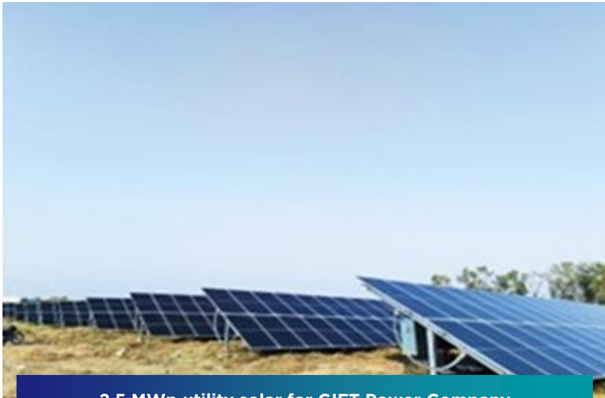
2.5 MWp utility solar for GIFT Power Company
