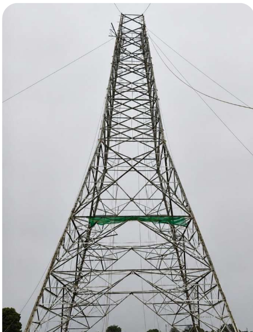
400 KV Madhya Pradesh
