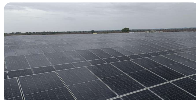
35 MWp Jalna, Maharashtra 1
