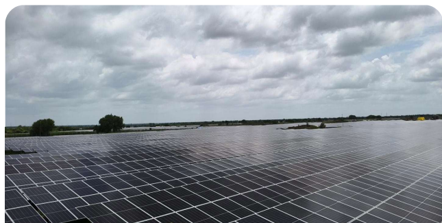
217.5 MWp Solapur, Maharashtra 1
