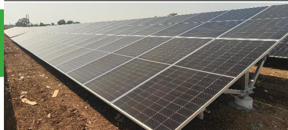
131 MWp Ground Mounted project at Nashik, Maharashtra
