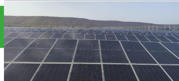
255 MWp Ground Mounted project at Neemuch, Madhya Pradesh
