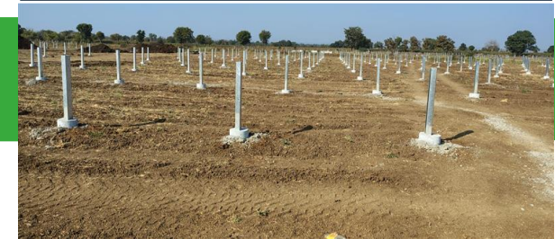
29.4 MWp Ground Mounted project at Yavatmal, Maharashtra
