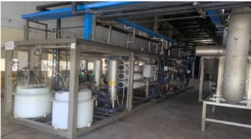
4th-Stage RO Installation – VFB
