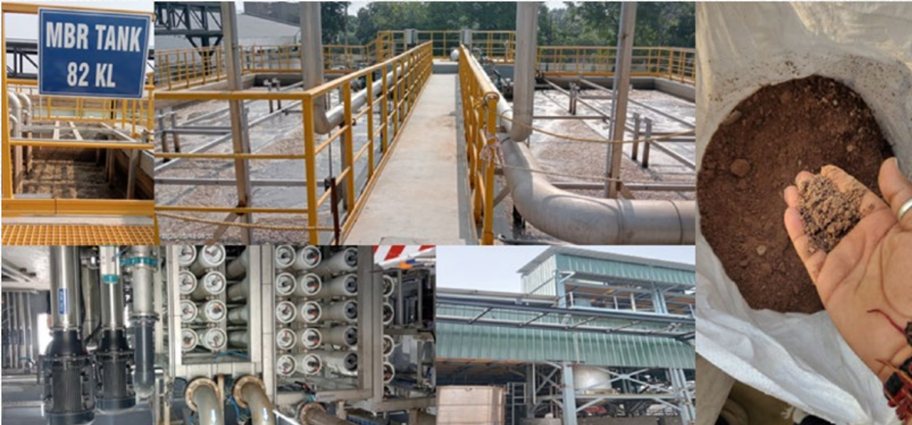
VSGM ZLD PLANT
