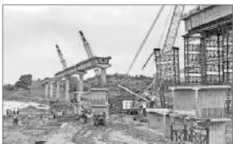
The site of Hamirpur bridge collapse on Friday.
