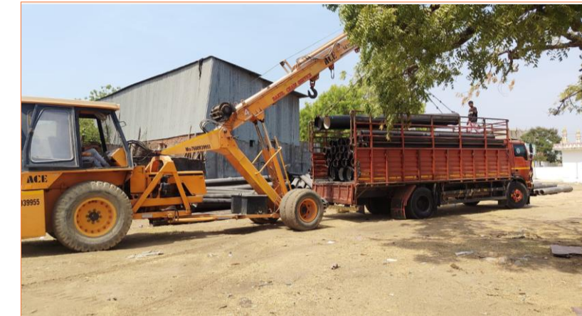
Project Name: Balasinor WSS and UGD Project Location: Gujarat Expected Completion: April 2027
