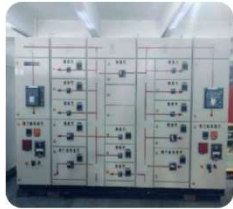
Motor Control Centres (MCC) Panel
