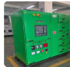
DG Synchronizing & Load Sharing Panels
