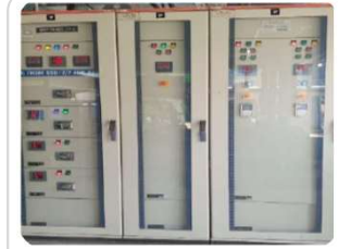
Variable Frequency Drive (VFD) Panel
