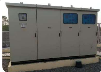
33kV RMG Panel
