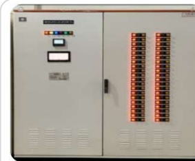
Power Distribution Unit (PDU)
