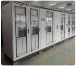
Power Control Centres (PCC) Panels
