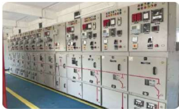
11kV/33kV VCB Panel (Vacuum Circuit Breaker)
