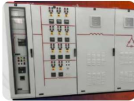
Automatic Power Factor Correction (APFC) Panel
