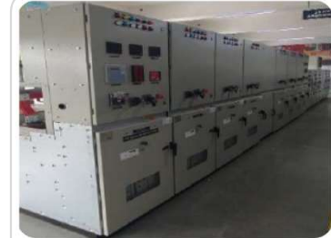
11kV DG Synchronizing & Load Sharing Panels
