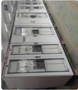
Power Control Centres (PCC) Panels
