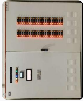
Power Distribution Unit (PDU)
