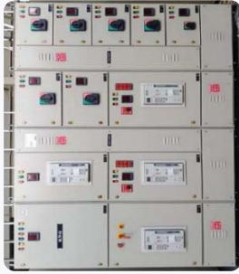
Intelligent Motor Control Centre (IMCC) Panel
