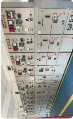
11kV/33kV VCB Panel (Vacuum Circuit Breaker)
