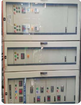
Variable Frequency Drive (VFD) Panel
