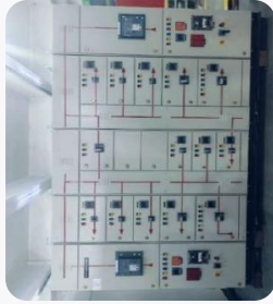
Motor Control Centres (MCC) Panel
