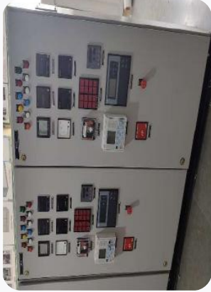
Control & Relay Panels (CRP) up to 33kV
