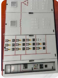
Automatic Power Factor Correction (APFC) Panel
