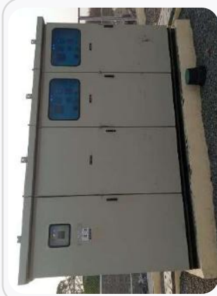
33kV RMG Panel
