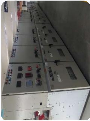
11kV DG Synchronizing & Load Sharing Panels
