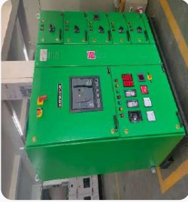
DG Synchronizing & Load Sharing Panels
