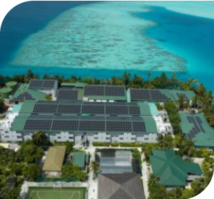
Solar installation, Maldives
