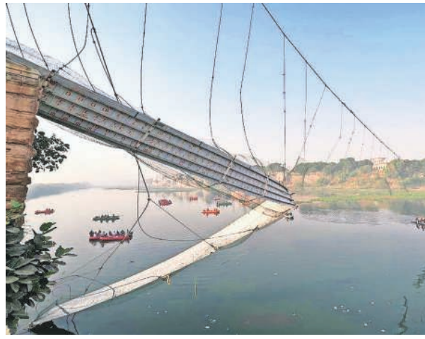
As many as 135 people were killed in the bridge collapse. File
