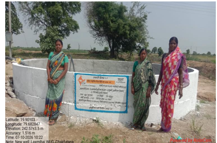
New well, Chak Futana, Pombhurna taluka
