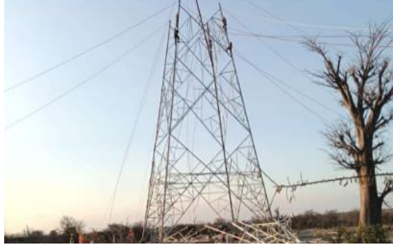
TaZa 400 kV D/C line, Tanzania Cross country project
