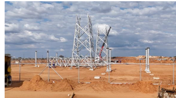
Mmamabula 400 kV substation, Botswana
