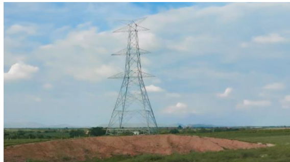
765KV D/C Dausa-Ghiror TL project, Rajasthan
