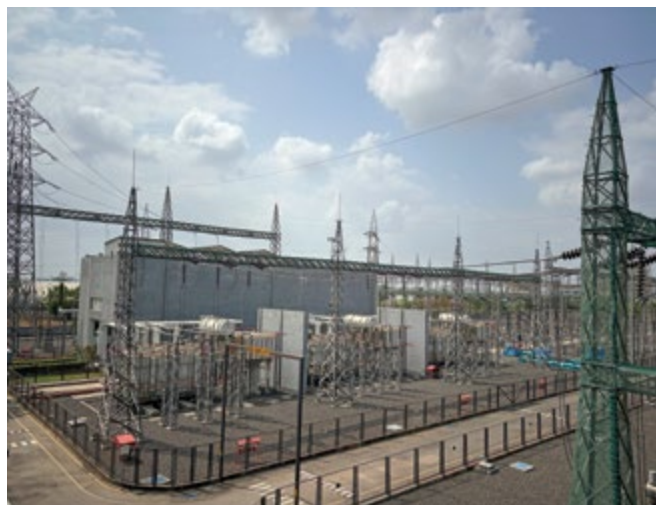
EHV Switchyard, Ahmedabad
