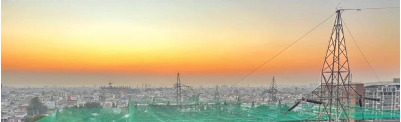
132 KV AIS Substation Switchyard, Ahmedabad
