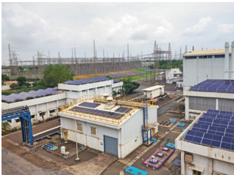
Solar Rooftop at SUGEN & UNOSUGEN
