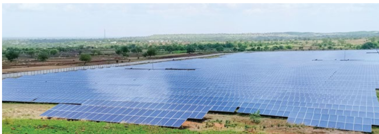
50 MWp Solar Power Plant, Maharashtra
