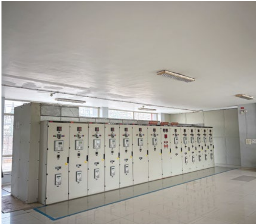
GIS Substation, Ahmedabad
