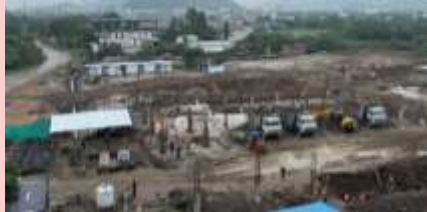
New plant – Unit 8
