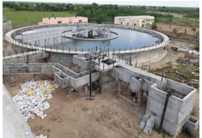
WTP at PHED Jawai Project, Rajasthan India
