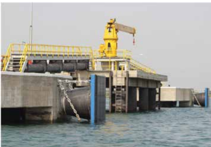
Mooring Dolphing and Pump House Ghana Water Company, Accra, Ghana
