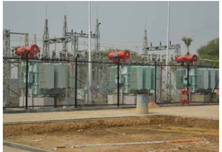
33/11KV Sub-Station at Banka, Bihar, India
