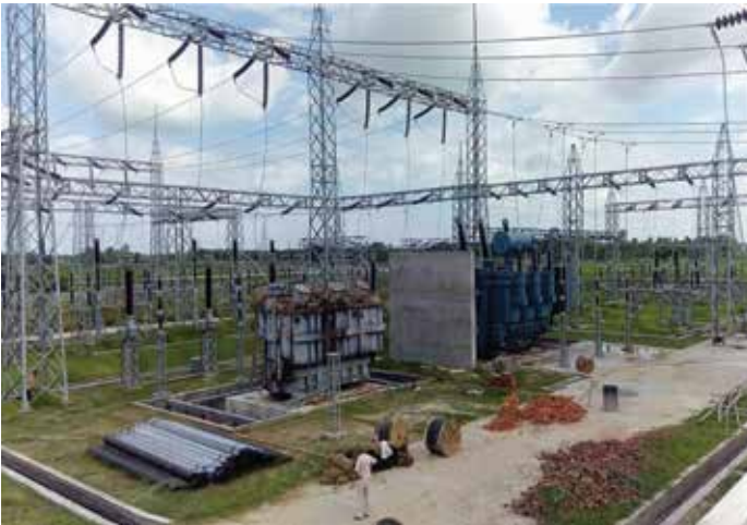
220 KV Substation UPRNNL, Bansi, U.P. India
