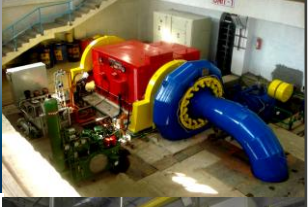
Hydro Turbine Generator & Site Installation
