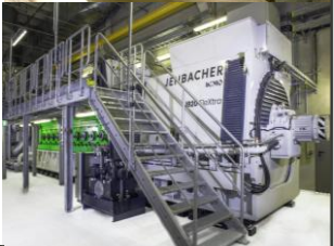
Gas Engine Generator & Site Installation
