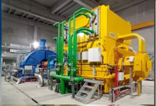
Steam Turbine Generator & Site Installation
