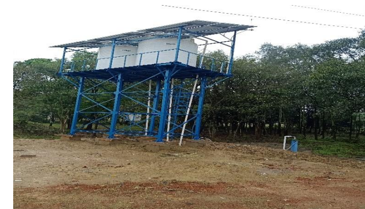
Solar power run drinking water system
