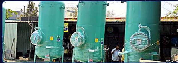
Nitrogen and air receiver systems
