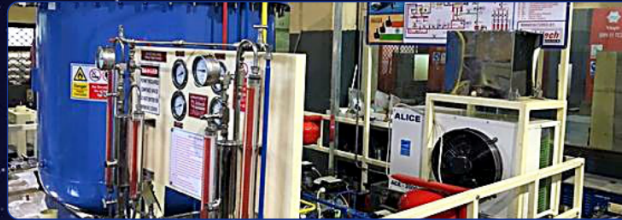
BRAHMOS fuel charging system
