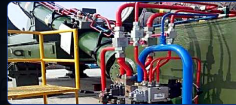
Power pack and cylinders, K-5 static launcher
