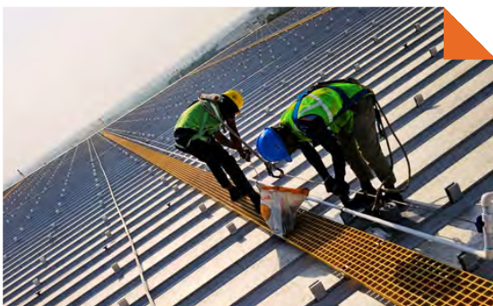
Topre India Pvt. Ltd. (1,173.70 kWp)
