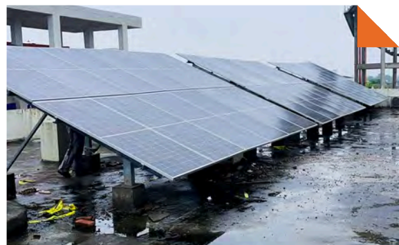
PEDA - Grid Tied Solar Plant (1470 kWp)
