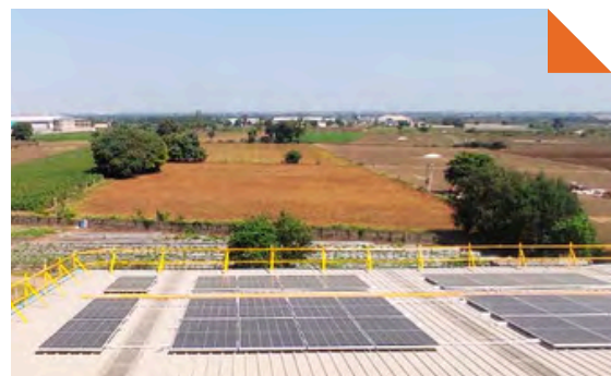
Max Power Engineers (49.5 kWp)
