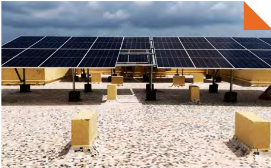
Shri Kolhapur Bhavan (49.5 kWp)
