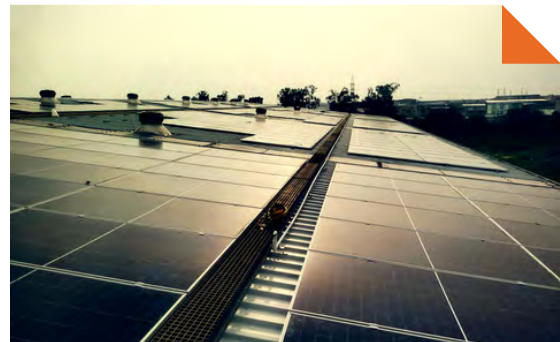
Embee Screens (378.36 kWp)
