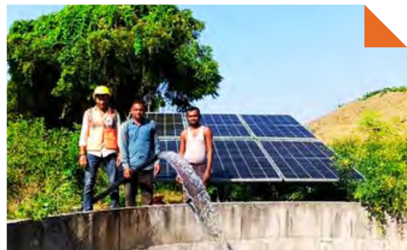
MSEDCL (1291 Nos. Solar Water Pump)
