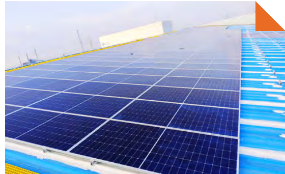
Ratnatris Pharmaceuticals (500 kWp)
