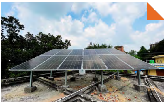
UPNEDA - Grid Tied Solar Plant (1400 kWp)
