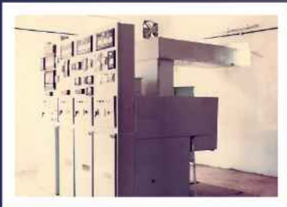
Indoor Circuit Breaker 12kV
