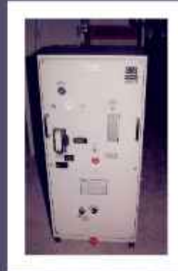
Circuit Breaker HHV12
