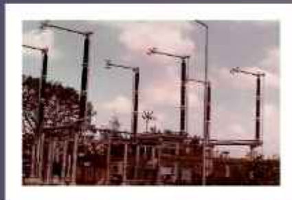
Center Break Disconnecter 420kV
