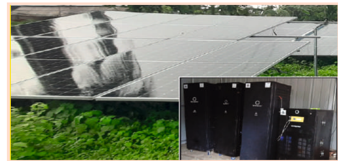
Capacity: 6 MWh BESS Location: Tripura
