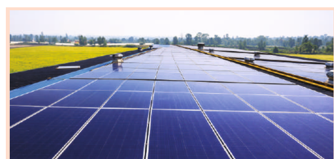
Capacity: 350 kWp Location: Globus Spirits Ltd. Lakhimpur, UP
