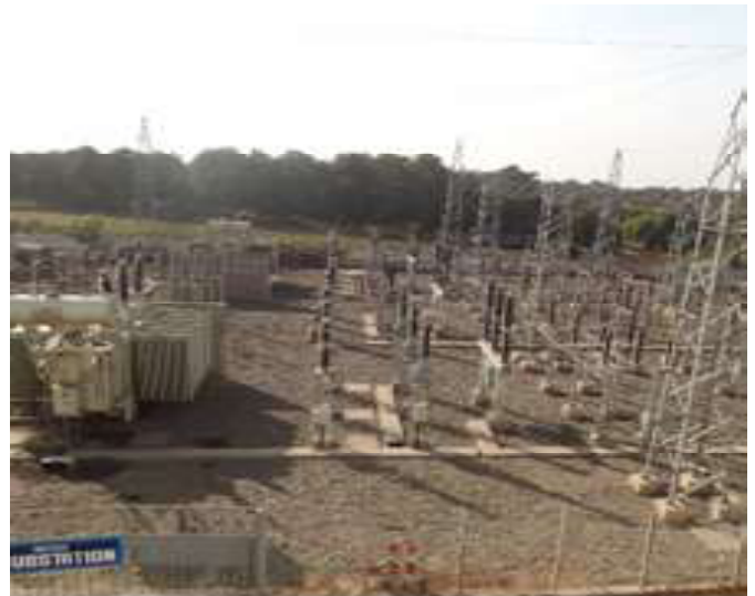
132KVA Sub Station
