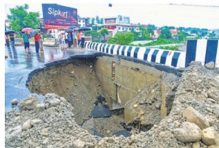
People gather after a section of a bridge caves in following heavy rainfall, in Dehradun, Uttarakhand
