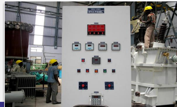
RTCC Panel Assembly
