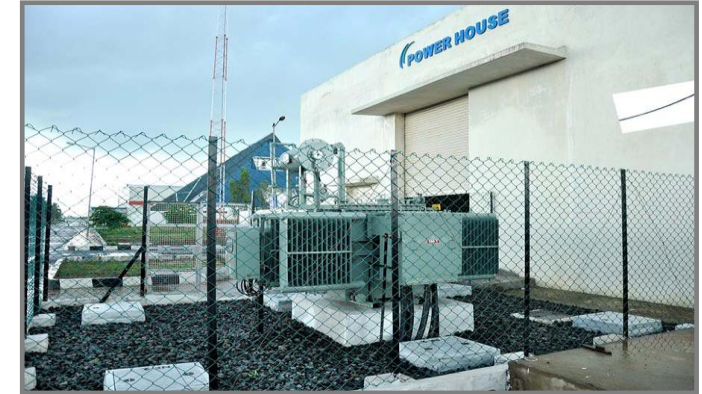
Project Name: Win Wind Energy Ltd Client: Vestas Location: Chennai Transformer Rating: 1250 KVA
