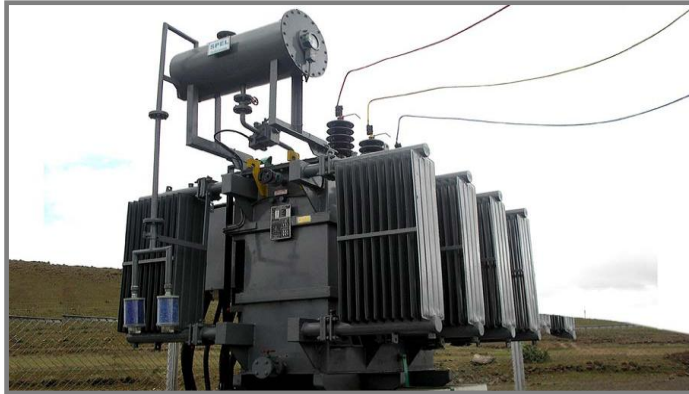
Project Name: Win Wind Energy Ltd Client: SIEMENS Location: Periapalayam, Chennai Transformer Rating: 1250 KVA
