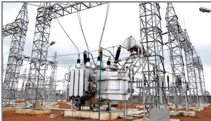
Project Name: 110 KV SS Client: TNEB Location: Alamathi Transformer Rating: 25 MVA
