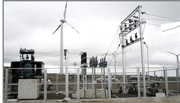
Project Name: Wind Mill SS Client: Vestas Location: Surandai Transformer Rating: 950 KVA
