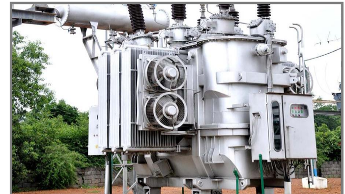
Project Name: 110 KV SS Client: TNEB Location: Gummudipoondi Transformer Rating: 16 MVA
