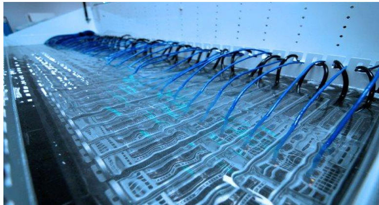
DATA Centre Cooling
