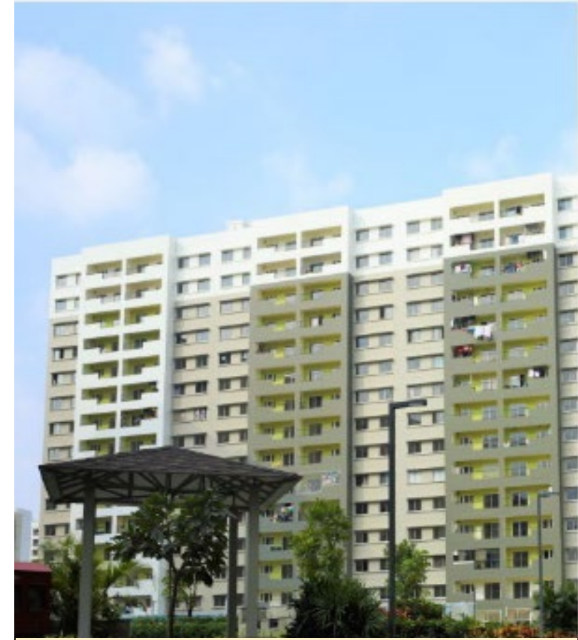
Wing 26 comprising 1 Tower of G+ 14 floors Total SBA completed in Q3-FY23 – 120,377 sft (120 units)
