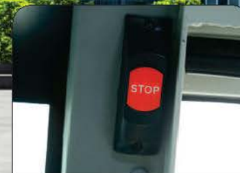
Individual Emergency Stop Switch
