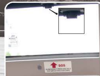
Emergency Stop Switches
