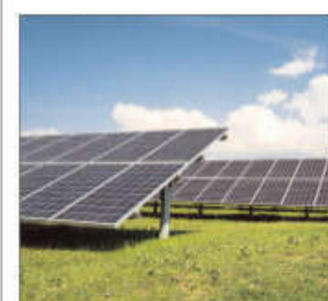
Solar capacity installed in 2023 was 8.3 GW, according to a Mercom report
