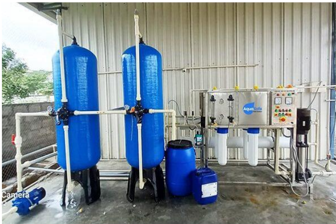
Installed 10 RO plants of 250 LPH at Gadag and Raichur for poor and underprivileged people
