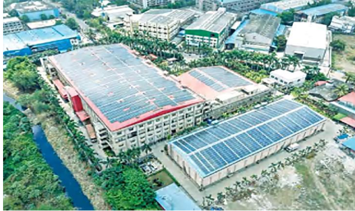
Solar Panel at our Plant
