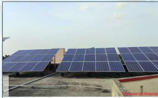
HPCL (offgrid) 250 kW
