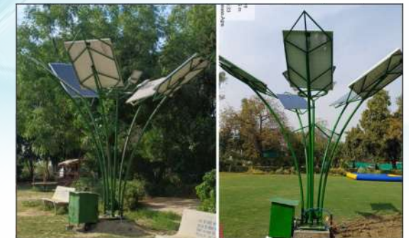
UPNEDA (OFF-GRID) 1kw off grid ( Solar Tree ) :20 sets
