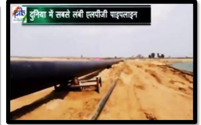
Kandla-Gorakhpur LPG Pipeline Solarizing a total of 158 sites on the country's longest LPG pipeline - spanning 2,757 Kms - from Kandla Port, Gujarat to Gorakhpur, Uttar Pradesh
