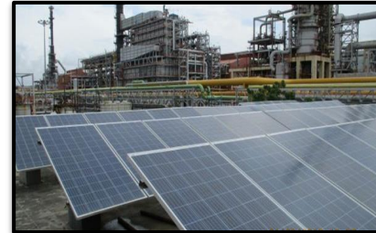
Rooftop Solar Project BPCL (Mahol Refinery)
