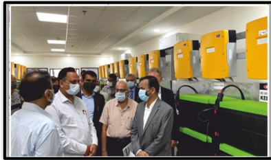
Shivalik Project Micro Grid Solar Power System Installed at Shivalik Grid in Delhi
