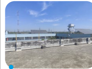
Sub District Hospital Tanakpur-100kW
