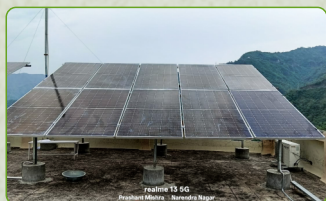
Glimpse of SSDH hospital Narendra Nagar-50kw
