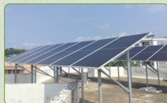
Glimpse of Sub District Hospital Tanakpur-100kw
