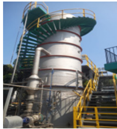
Zero Liquid discharge plant in SLW, Kolkata.
