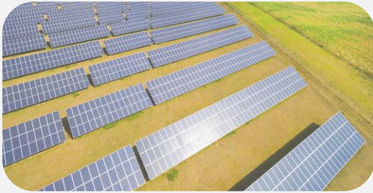
Ground Mounted Projects
