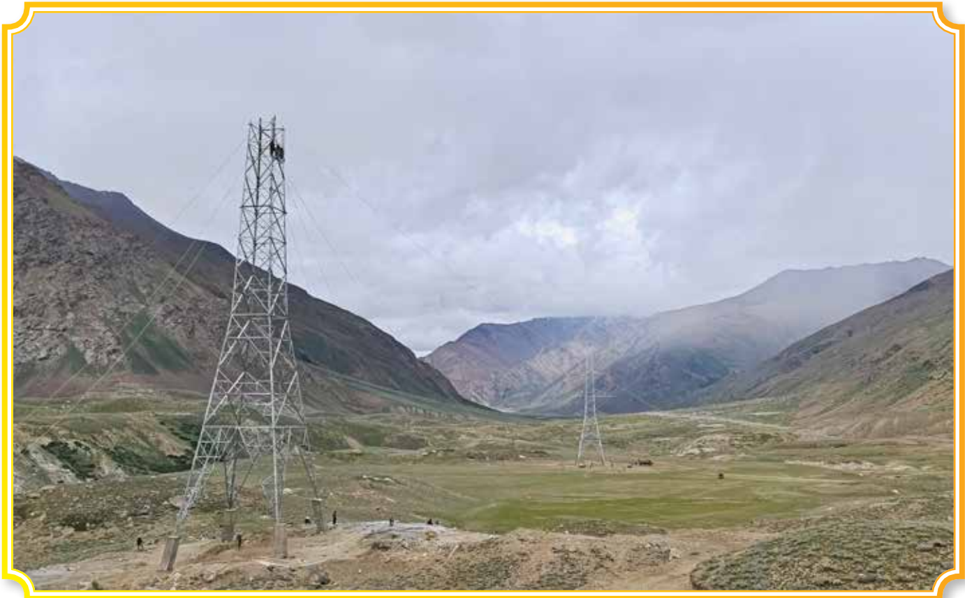
220kv Single Circuit Transmission Line from Drass to Padum on Double Circuit Tower at Kargil, Ladakh being implemented by RECPDCL
