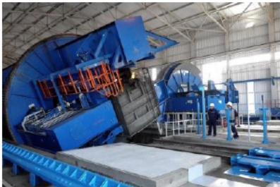
Wagon Tiplers, Conveying System (Raw Material Handling etc.)
