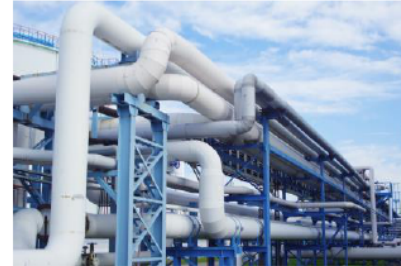
Fabrication and erection of Piping of such as CS/ SS/ Alloy steel including above ground and underground
